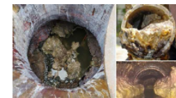
Clogged pipe Caused by improper grease disposal
